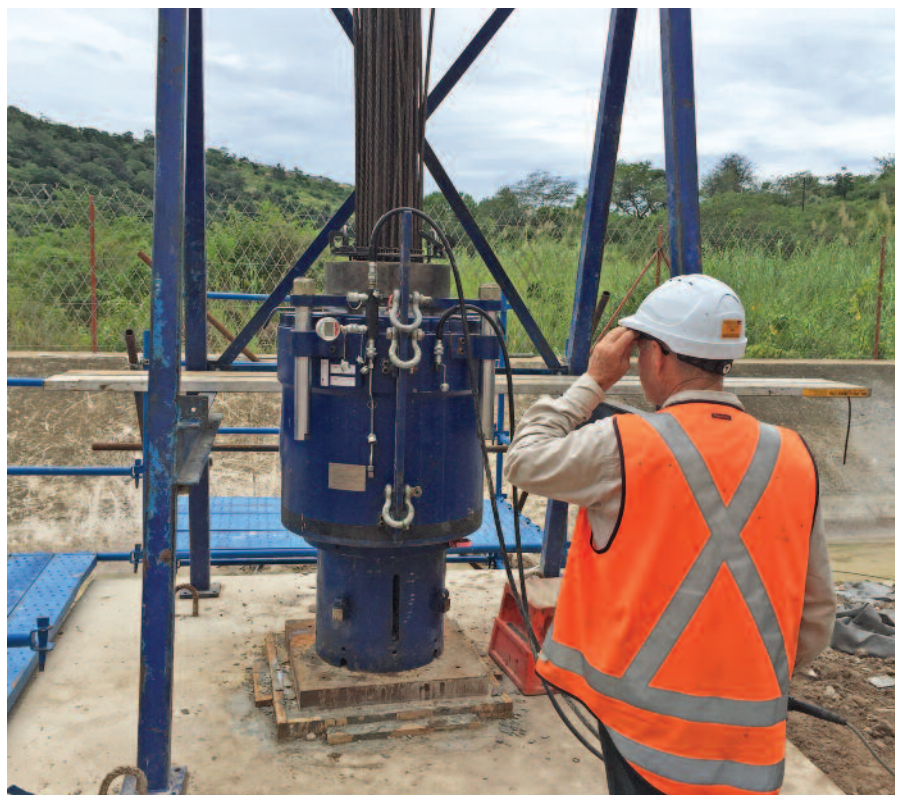
Figure 9 61 Strand test anchor stressed with a 3372 kips capacity stressing jack at Hazelmere dam.
